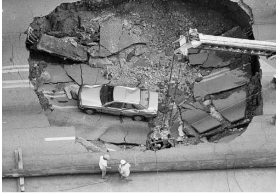
Figure 3 ▶ When land overlying a cavern collapses to form a sinkhole, human-made structures, such as this highway, are often damaged.
