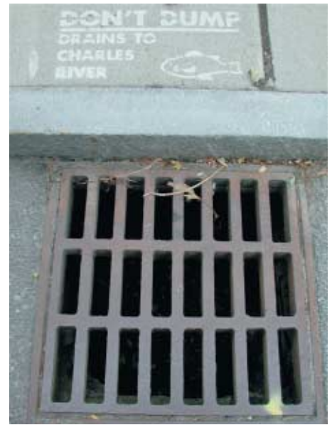
Figure 5 ▶ Water that enters this drain runs off into the Charles River and surrounding aquifers in Massachusetts.
