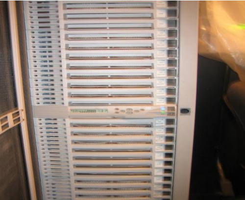
Figure 51: Dimmer rack, open
