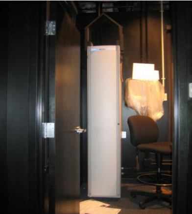
Figure 52: Dimmer rack, shut
