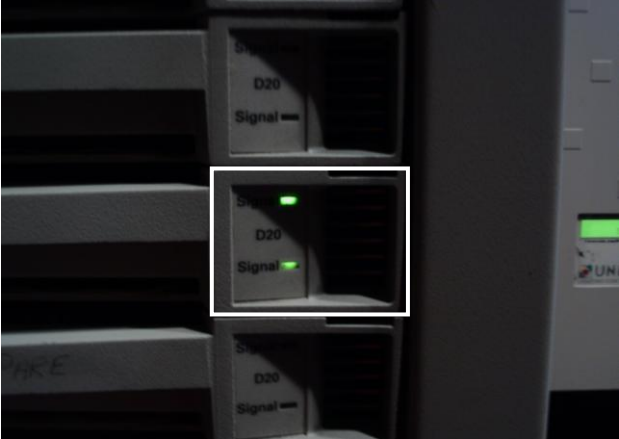
Figure 54: An active dimmer card (center)
