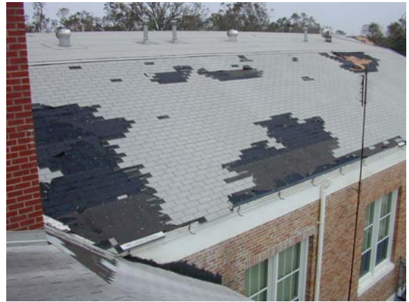
Charlotte Hyatt Elementary received extensive roof damage from Hurricane Katrina.
